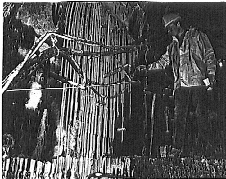
Photograph 5. Resin flowing back into Gallery through horizontal joints from points of injection 3m distant.
