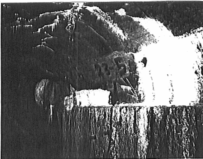
Photograph 1. Water inflow into Lower Gallery from large diameter chimney drain (left). Note also calcification on walls from seepage through horizontal joint.
