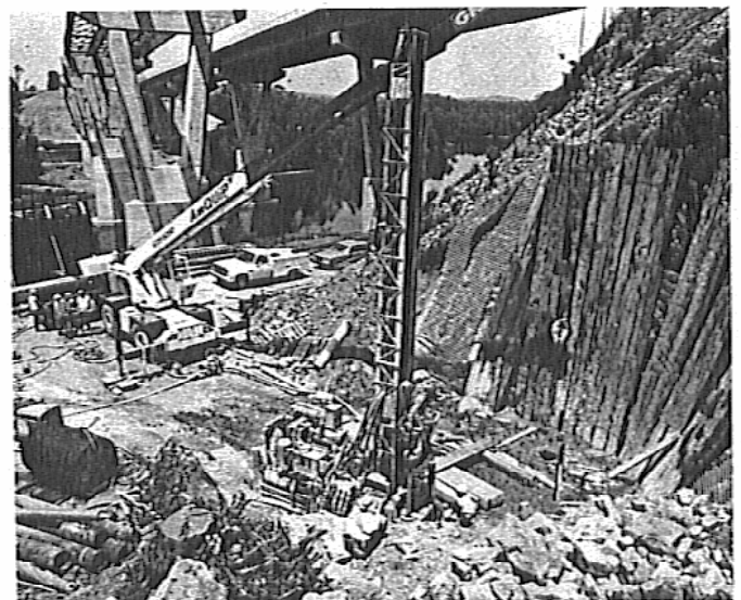
Diesel Hydraulic Track Drills for Nicholson Pin Pile Installation I-78 Bridge, Warren County, NJ between New Jersey and Pennsylvania.
