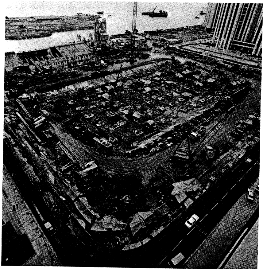
Overall view of the Icos Vibro site. Blasting took place in the area at left of photo.
