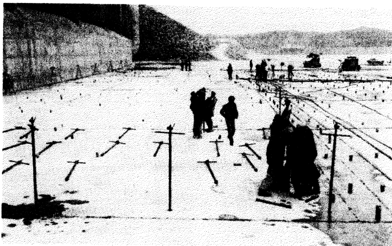
Fig. 6. Mechanical grout packers placed in drill holes in preparation for panel lifting
