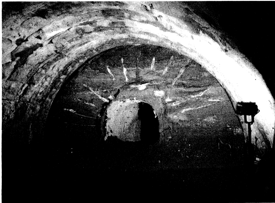
Figure 16 View of pilot and full bore, showing end of jet grout columns, and radial tubes à manchette. Milano Metro Line 3.
