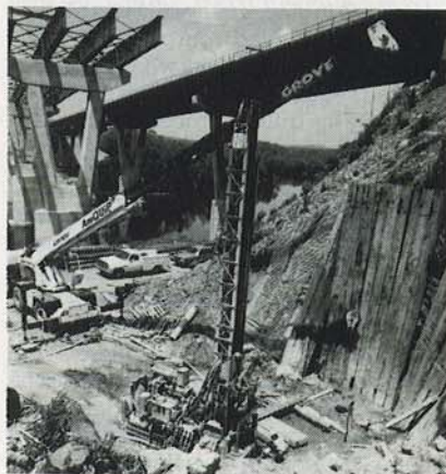
Pic. 5. Installation of minipiles to underpin bridge pier 6E over the Delaware river. Warren County, NJ.
