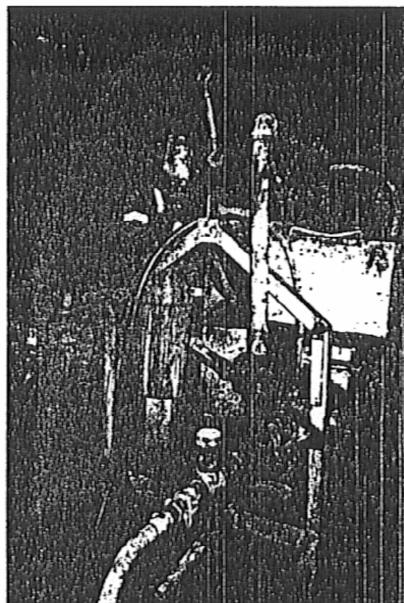
Photograph 4. Mixer pump unit where bagged cement (left) was added to standard Mine slurry (top pipeline, left).
