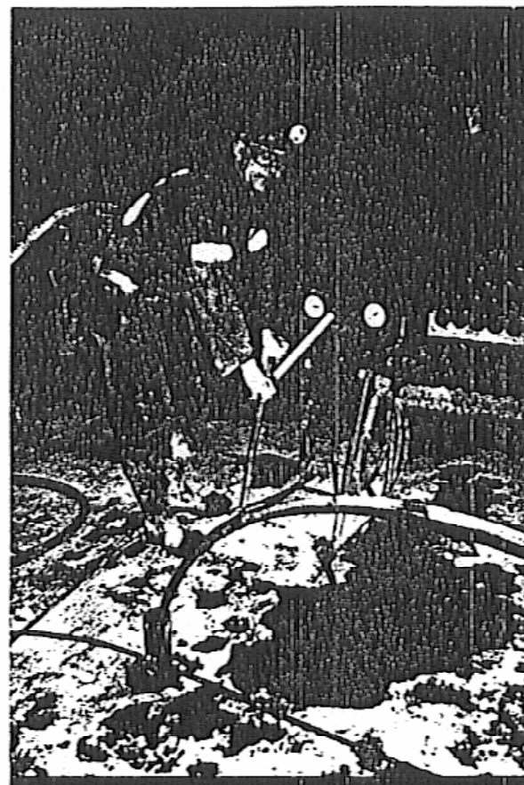
Photograph 5. Hand pump used to inflate packer attached to flexible groutline placed in MPSP pipe (left foreground).
