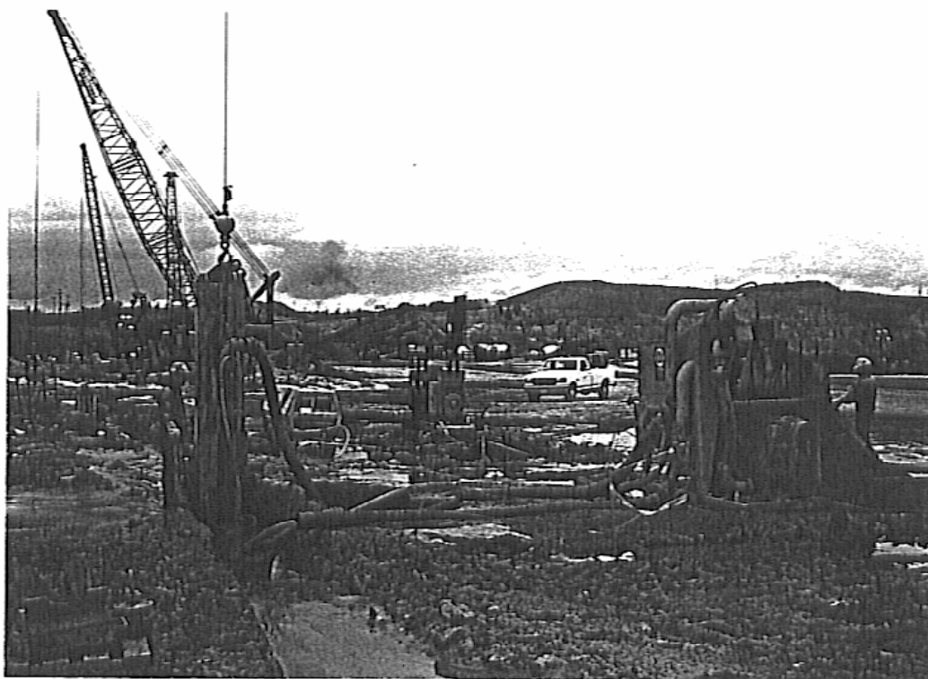
Photograph 4. Desanding of Secondary panel prior to concreting. End stop shown at far end of panel.
