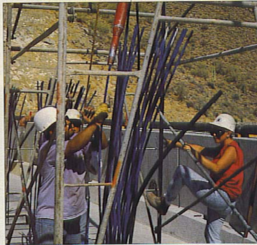
EVERY ARCH TENDON WAS COMPOSED OF 22 EPOXY-COATED STRANDS, EACH 0.6 IN. IN DIAMETER. DESIGN LOADS AVERAGED ABOUT 665 KIPS.
